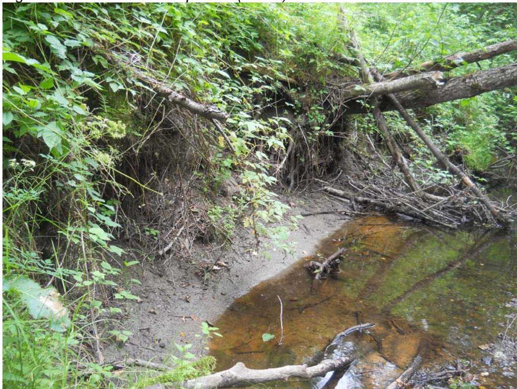
Figure 11 Sapement important en berge (S-279)
